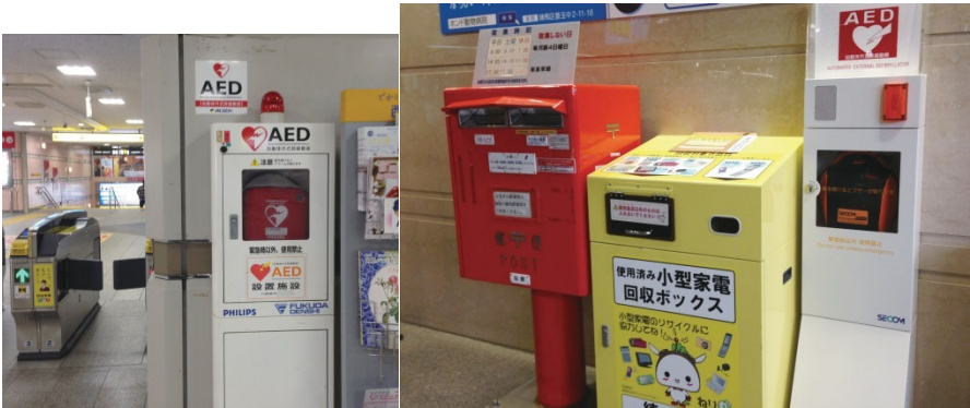
Fig. 5.7 Examples of Installed AED Boxes (Ministry of Health, Labor and Welfare, 2015)
